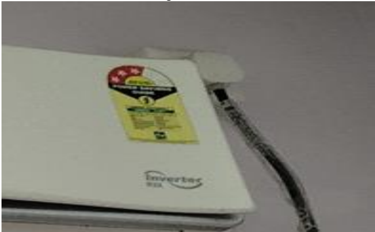
Air Conditioner with 3 Star Energy Rating at BMS Ground Floor Lab
