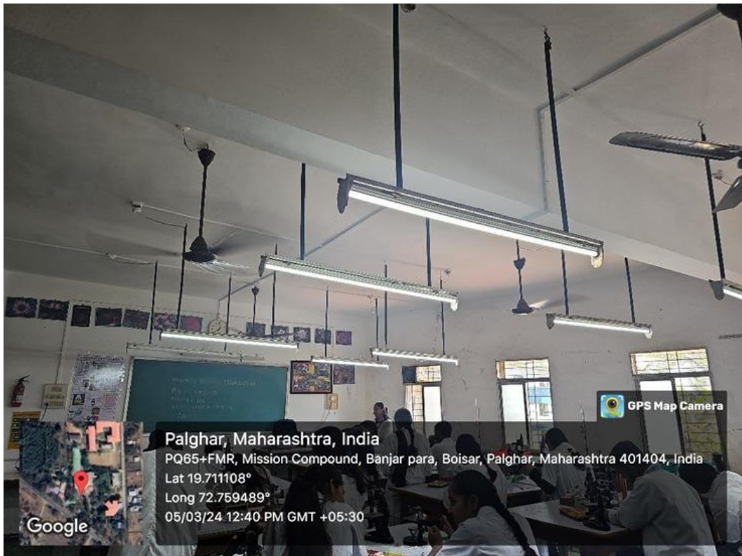
Main Building Botany Department Labs equipped with energy saving led tube lights.
